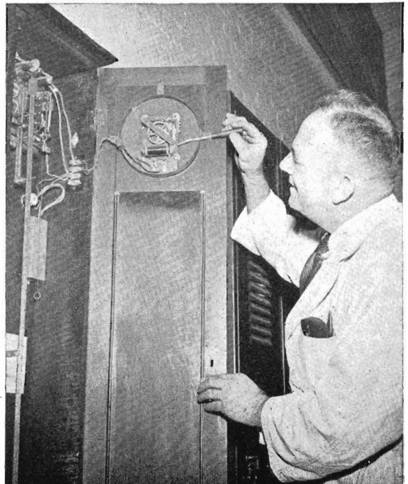
A mechanic adjusts the master electric impulse clock which controls the other clocks in Head Office. Electric impulse clocks, which are also installed in the Flinders-st. offices and Newport Workshops, are serviced by staff from the Depot.
