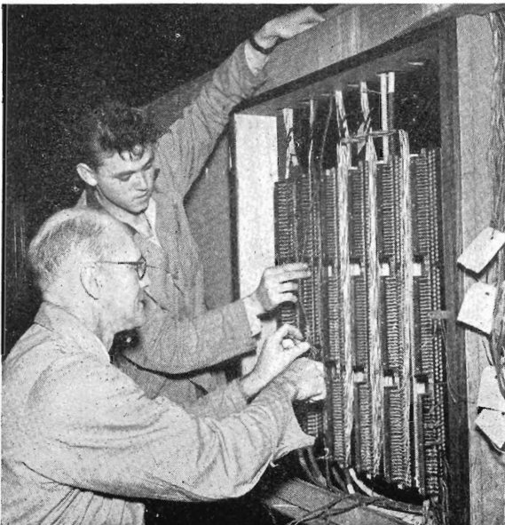
Electrical mechanic at work re-locating dictograph cable terminations in an altered section of Head Office. Alterations to offices involve considerable work on the internal communications system. On this particular job fourteen cables of 52 wires each had to be dealt with.
