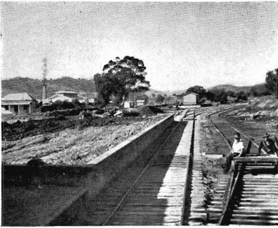
Above New Tallangatta station and stock-yards (left) under construction at Bolga—site of the new Tallangatta township after the old town is submerged by the increased Hume Dam capacity.
