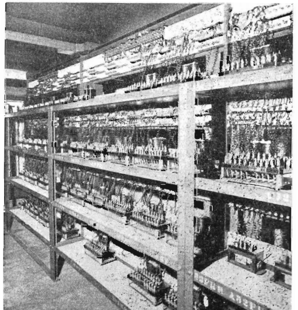
A relay rack used for relay interlocking. This shows a section of the intricate mechanism operated from the control panel in the signal box.
