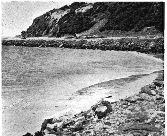
Rubble bank below Battery Point to give rail access to the new shipping berths.
