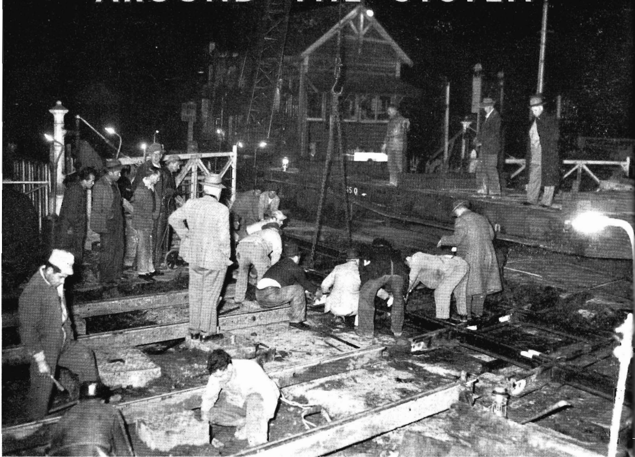
TRACK WORK : Way and Works staff must carry out some types of suburban track and bridge work after the last train has run, to avoid interference with traffic. Recent case was the placing of a new tramway square at the Burke Road crossing, Gardiner. A special train, with a steam crane, was used in the operation. The foundations were laid the previous week-end.
