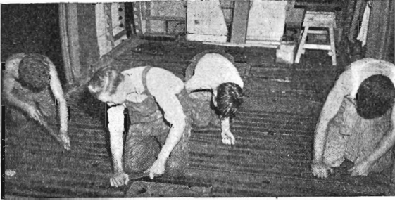
Preparing the steel floor for the cork covering. On the cork are placed masonite sheets and rubber, a combination that provides good insulation and resists wear.
