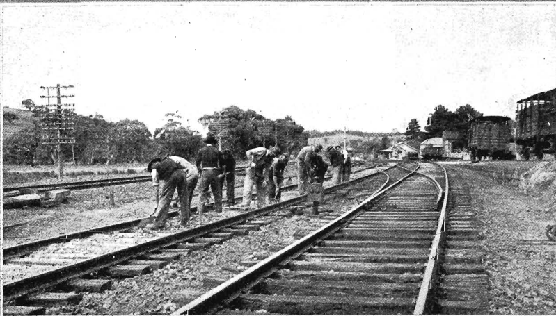
MAINTENANCE: The programme of track maintenance is being pressed forward. Track gangs are here seen ballasting near Kilmore East.
