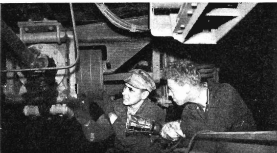
Adjusting the tension of the main drive belts of an air-conditioned car.
