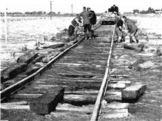
Track and bridge gangs starting the day's work in the Niemur area. Water was 10 inches above the rails.
